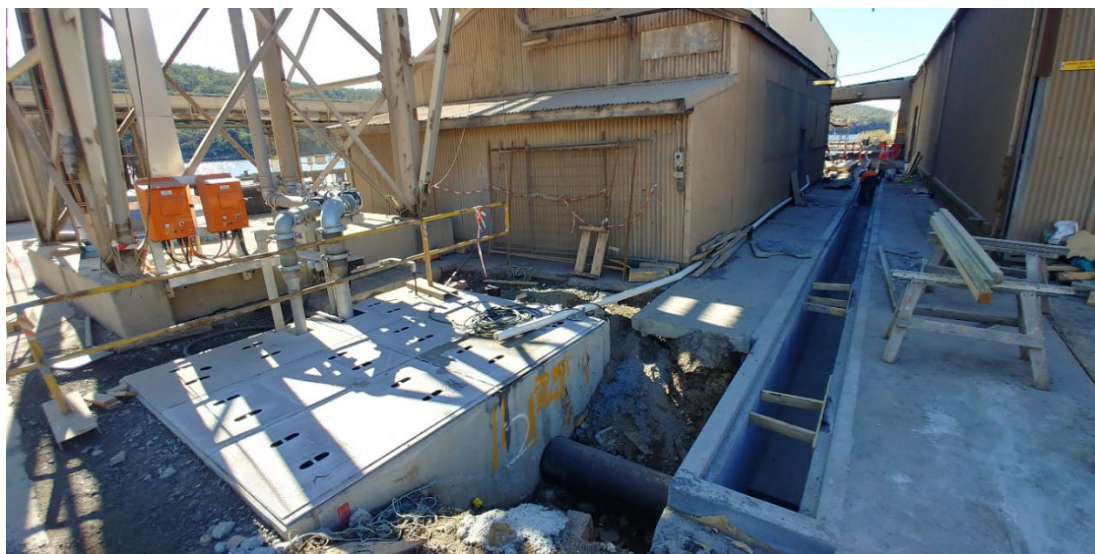
Figure 2-8 Image of one of the stormwater pits, and drains installed at the Wharf
